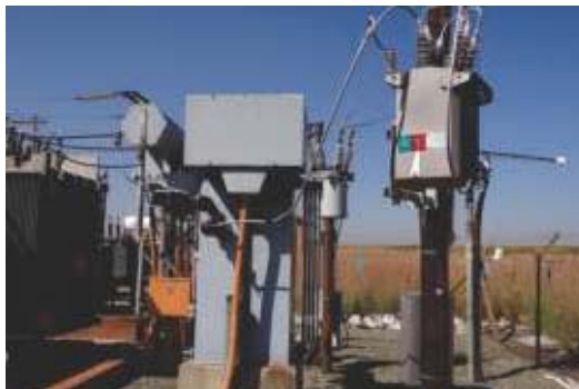
Fig 3: Practical installation of a NEC neutral breaker
