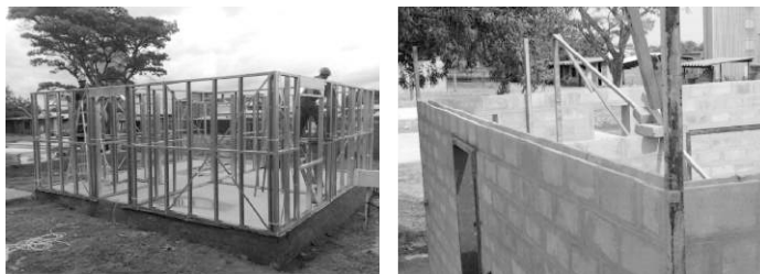
Figure 1: Illustration of the different construction technologies of light-weight highly insulated (left) and heavy-weight high thermal mass.
