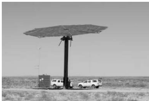
Figure 2: Eskom Heliostat experimental system for concentrated solar power generation
