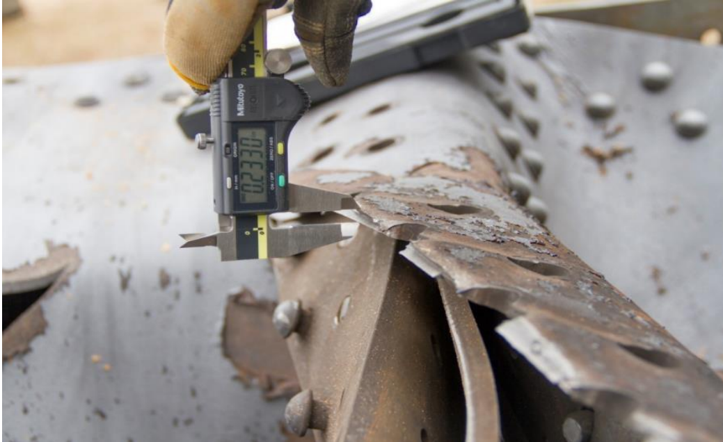
Fig. 3-3: Significant Necking of Riveted Plate Material (from Crane et al., 2015)
