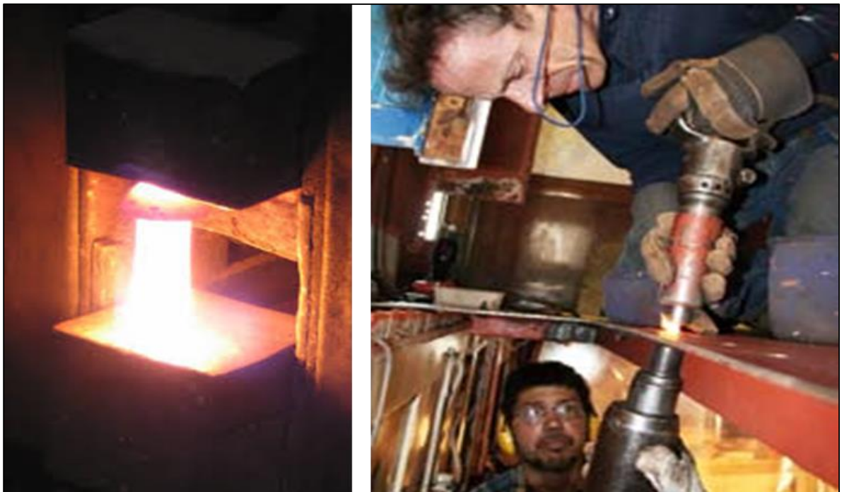
Fig. 2-1: The Riveting Process: the rivet heating (left); the rivet head forging with pneumatic hammer (right) (from www.efd-induction.com )
