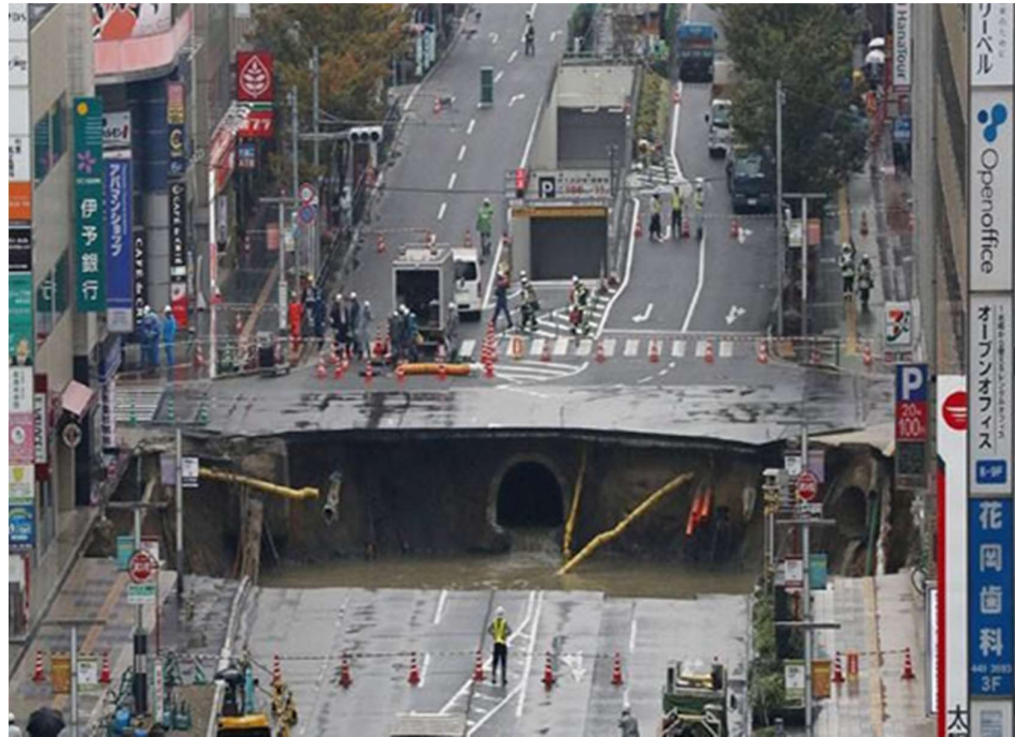
Figure 1. 4 Fukuoka sinkhole (Levy 2016)
