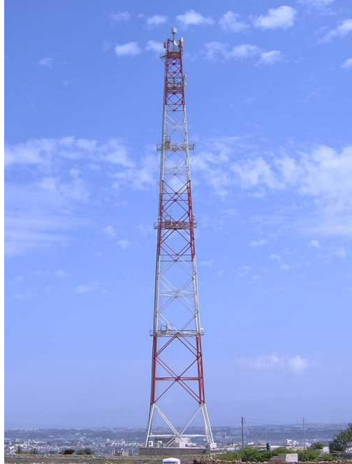
Figure 2 - An example of a radio transmission tower
