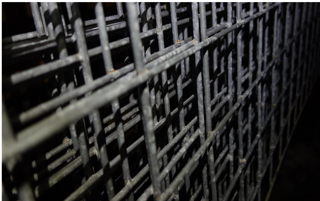
Corroded welds which can affect the screen's retaining capacity
