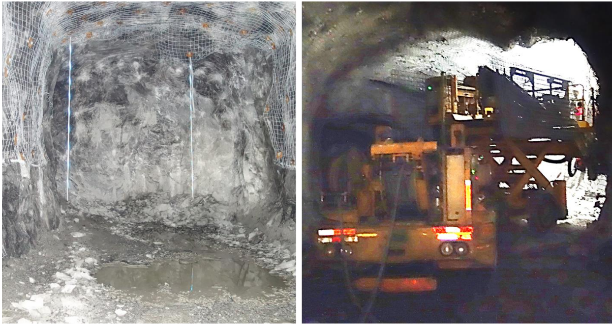
Figure 5.3 Left: Typical unbolting round; Right: MacLean bolter in an irregular heading Bolting under sandfill (hydraulic cemented fill) is only completed with the Boltec at Mine C, other types of rounds are shown in Figure 5.4. The Boltec is typically used in areas that require Swellex and irregular or sandfill rounds that cannot be bolted with the MacLean bolter such as irregular rounds.
