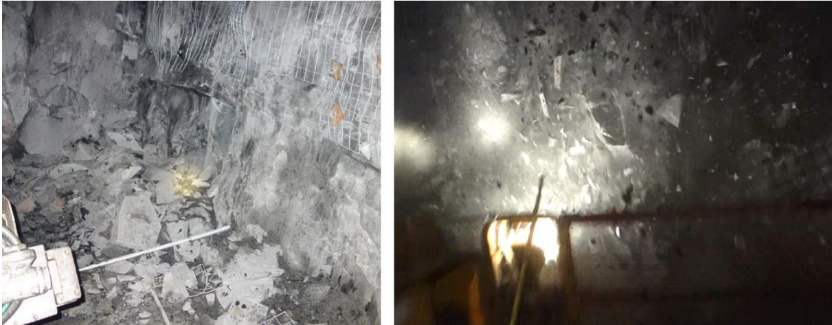
Figure D-4 Left: Rock ejected from lower wall during bolting; Right: Rock is ejected from the upper corner of a drift during a strainburst
