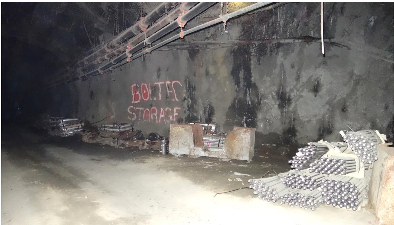
Boltec supplies storage at Mine C
