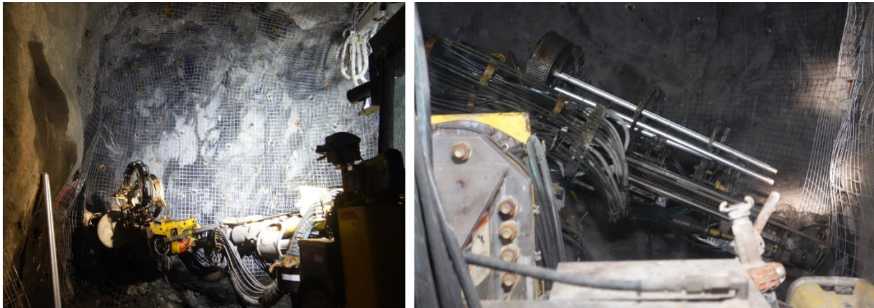
Figure 6.6 Left: face bolting contributes to cycle time Right: lower wall bolt installation contributes to increased cycle time
