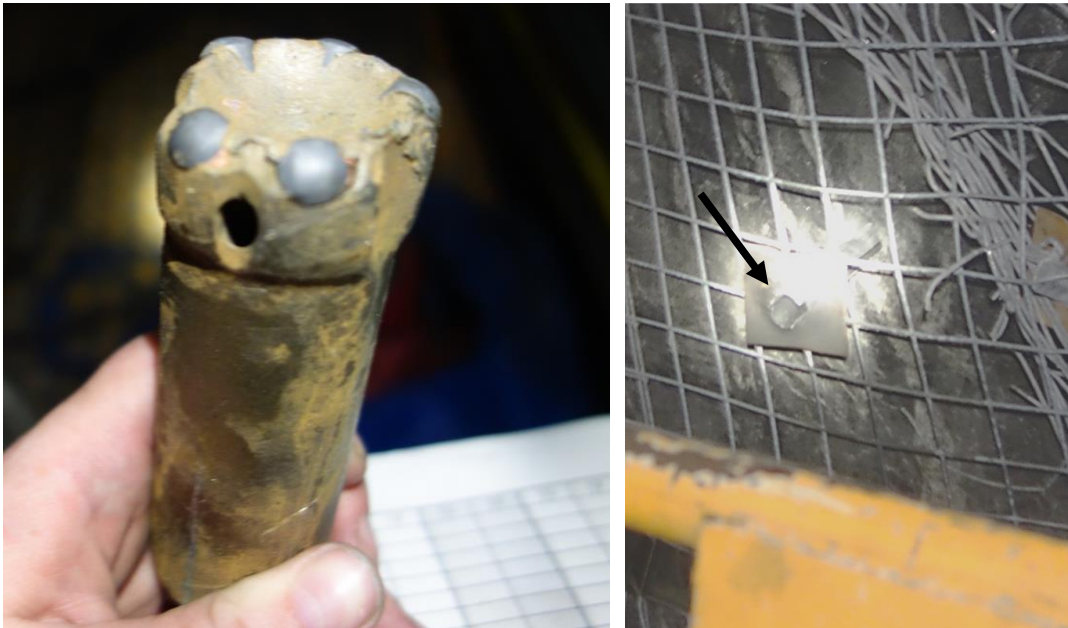
Figure 6.2 Left: Unusual bit wear on re-sharpened drill bit after drilling two holes, the drill bit passes the bit gauge test; Right: Split Set ring has fallen off a bolt due to long drive times during installation
