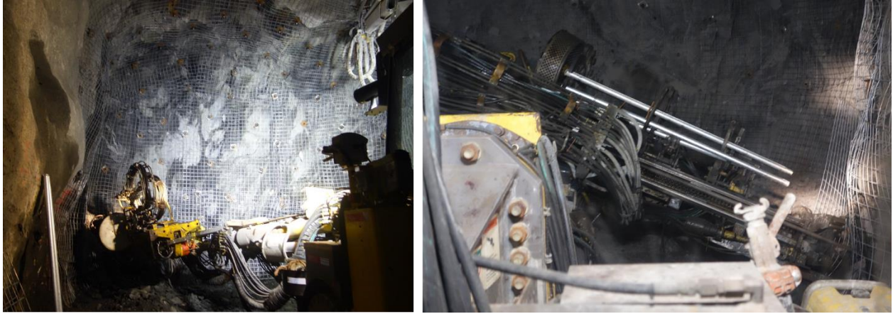
Left: face bolting contributes to cycle time Right: lower wall bolt installation contributes to increased cycle time
