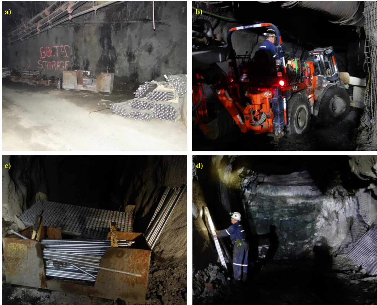
a) Boltec supplies storage on the 2340 m level b) Transportation of Boltec supplies with forklift c) Storage bins next to Boltec d) Operator “gearing” heading by leaning bolts and screen on drift walls
