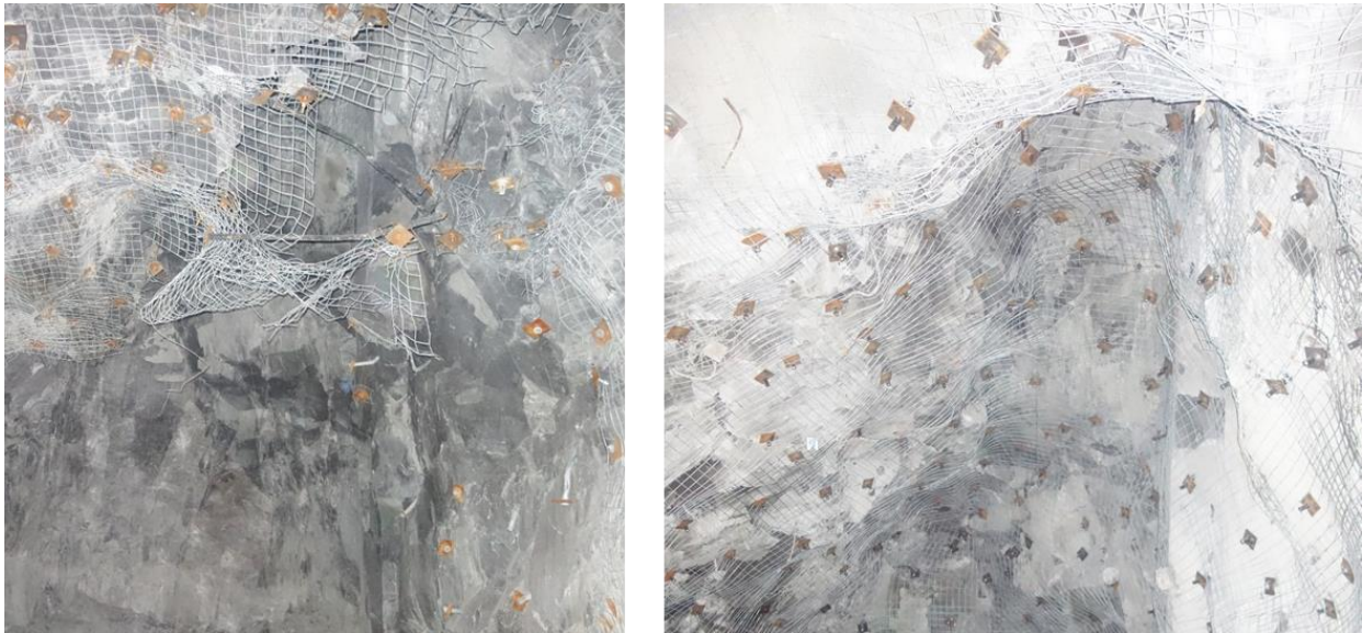
Figure D-5 Left: Wedge failure in a drift; Right: Installed bolts after wedge failure reconditioning
