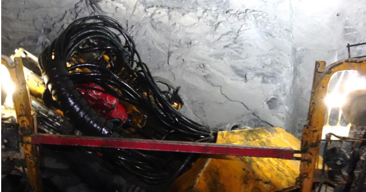
Damaged hoses on base of drilling tool (drilling tool is pointed downward)
