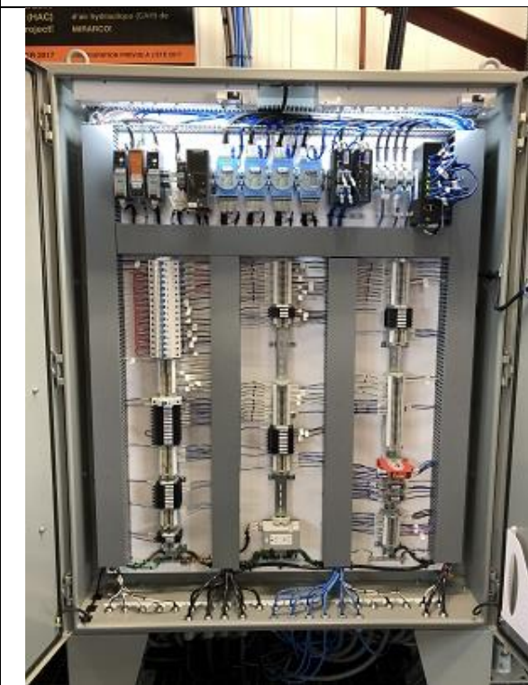
CP1 – Control panel (Open)
