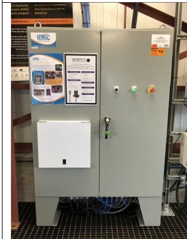
CP1 – Control panel (Closed)
