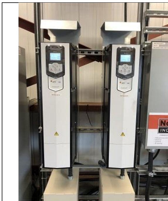
VFD1, VFD2 – Variable frequency drives
