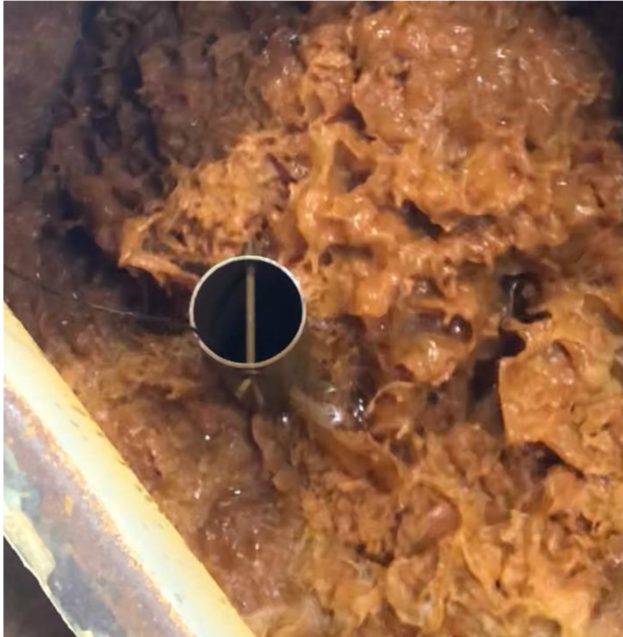
Figure 7: Water ‘sloshing around’ in the forebay tank during operation.
