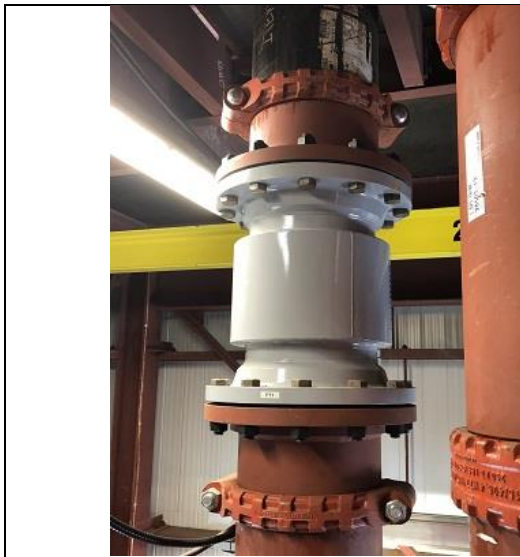
FT1 – Water flowmeter
