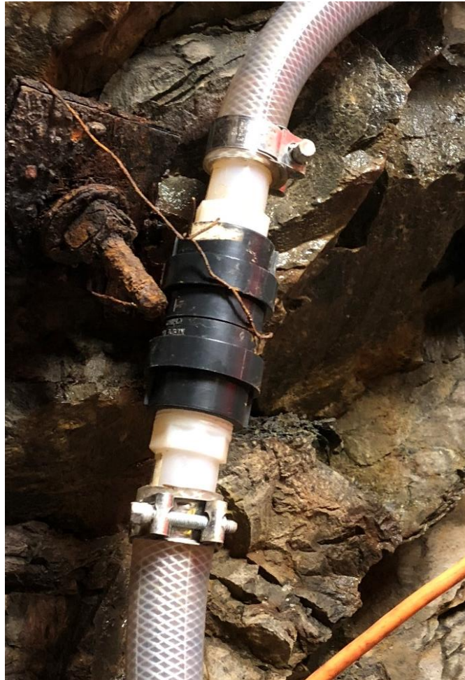
Figure 40: Check valve installed on the sump pumps drain line, also indicated on Figure 39 with a green checkmark.
