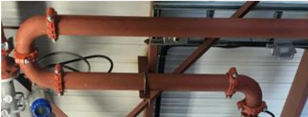
Figure 28: Compressed air line showing some of the Victaulic couplings.
