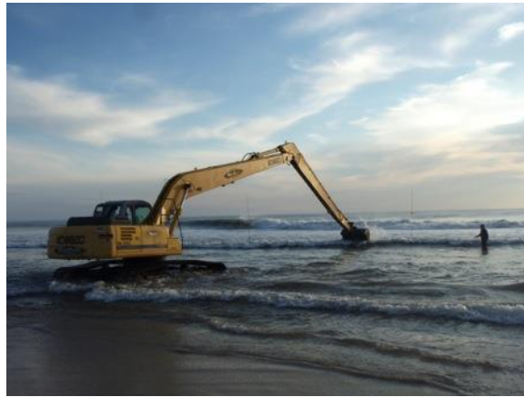
Figure 2.1. Backhoe excavating a hole in the inner surf zone near Duck, NC at low tide.
