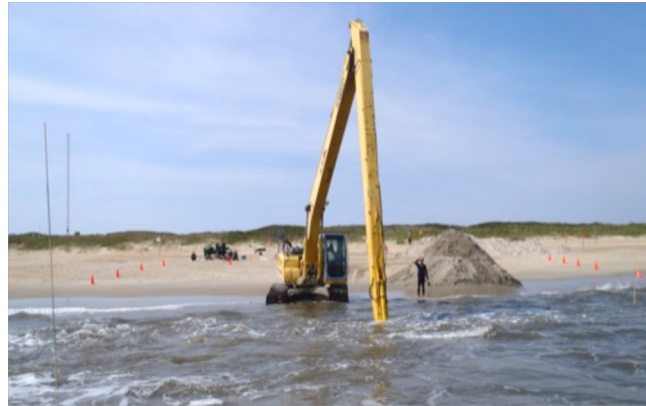
Figure 1.2. Photograph of equipment used to excavate holes in the inner surf zone near Duck, NC in 2010. The pile of sand was removed after the hole was excavated.
