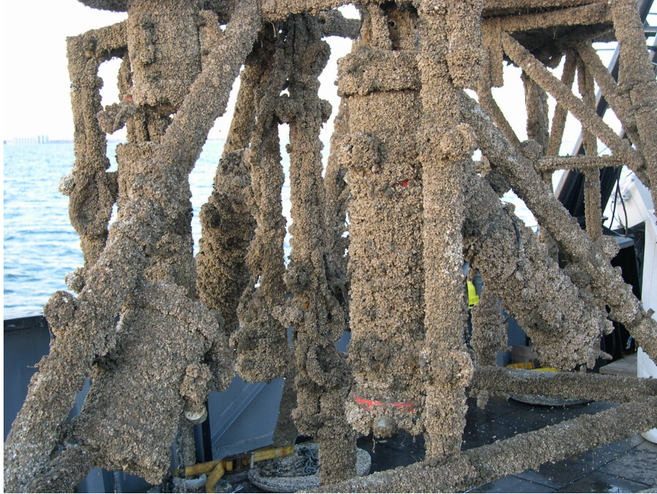
Figure 4-1: After several months of exposure to marine life, heavy biofouling develops on offshore structures. Such biofouling is an obstacle to thorough inspections and non-destructive testing [54].
