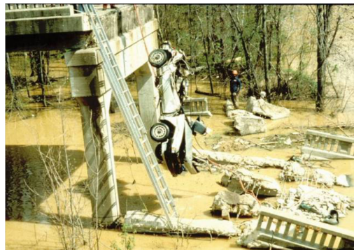
(b) US51 bridge collapse, Hatchie River, TN, 1989 (USDOT)
