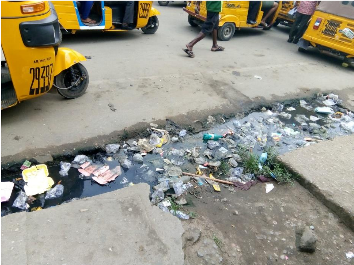
Picture 3: A Refuse-blocked gutter near Aba Main Park [Credit: Researcher]
