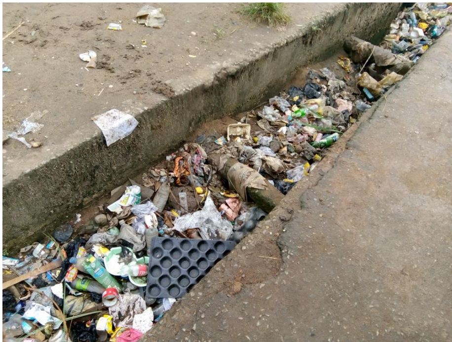
Picture 6: A Gutter/Drainage along Aba-Owerri Road (Near Star Paper Mill) [Credit: Researcher]
