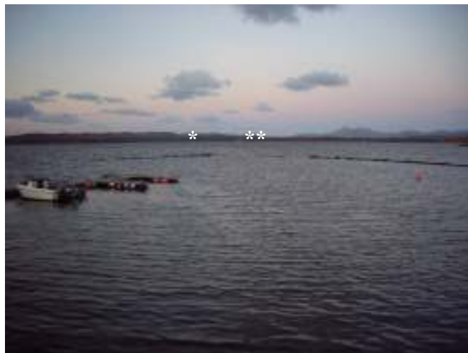
Figure 118 Shows the holes in the break water towards the North East corner (indicated by * and **). The hole at the corner being down to the beach level and the second being slightly shallower.
