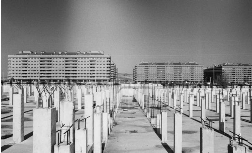
Figure 3: El Quiñón, Seseña: apartment blocks lie empty and the foundations for others have been abruptly abandoned (Photograph: Joshua Aylett, 22 October 2015)
