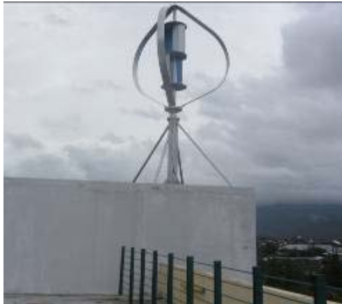
Figure 4-9: Non-operational vertical axis wind turbine in Banda Aceh
