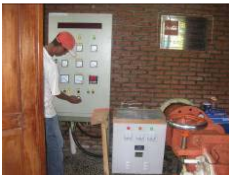
Figure 4-5: A community member operating Jantho micro hydro plant
