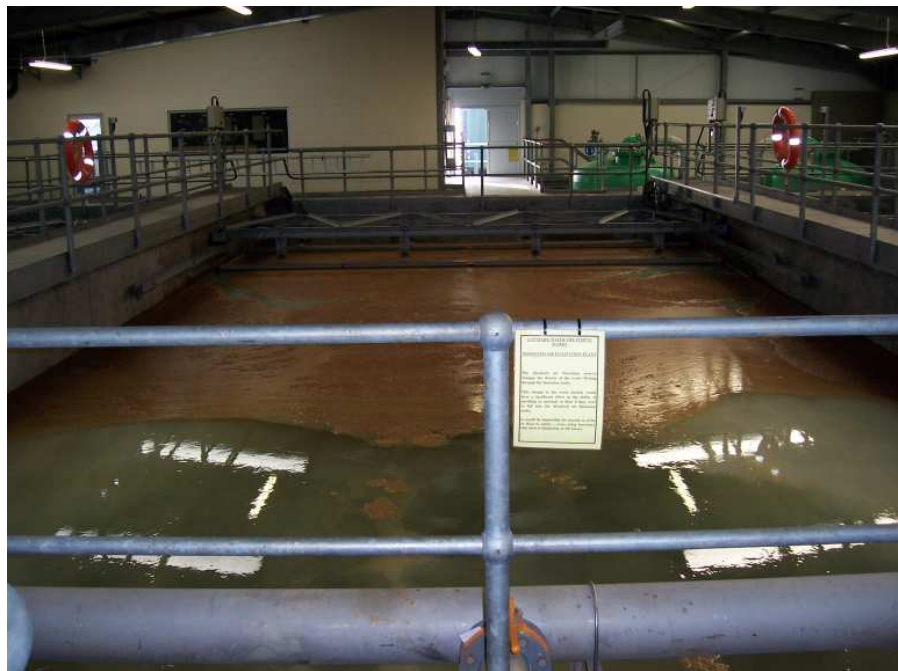
Figure 1-8. The water draw-off tower at Glenfarg reservoir, with the dam in the foreground (top). One of three DAF tanks at Glenfarg water treatment works with surface sludge clearly visible (bottom).
