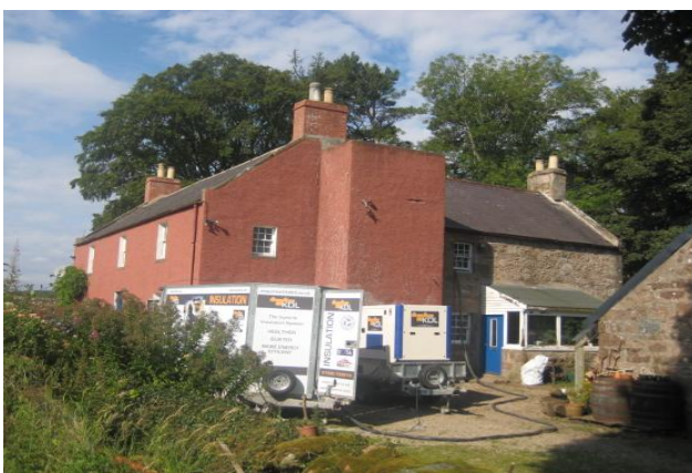
Figure 1. View of the house during the insulation process For the Scottish context this research/experiment will concentrate on existing load-bearing masonry construction with internal plastered lath lining.
