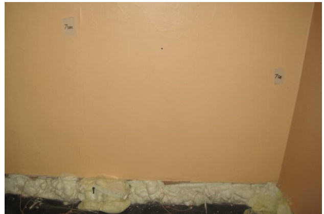
Figure 14. Leak of the foam at the bottom part of the wall
