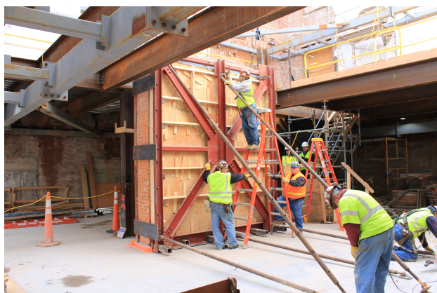
Figure 6 Structure being moved by crane, showing the left side cut of the brick supporting wall. Photo: ©President and Fellows of Harvard College, photographed by the Straus Center for Conservation.
