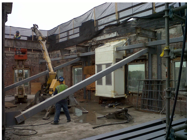
Figure 5 End of the World in its protective housing after removal of the roof of the building. Photo: ©President and Fellows of Harvard College, photographed by the Straus Center for Conservation.
