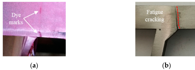
Figure 2. Typical cracking pattern: (a) Crack identified by DP checks; (b) Macro-section of the cracked joint.
