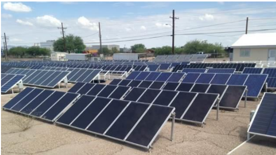
Fig. 2. Strings of PV modules at TEP/AzRISE test yard in Tucson, AZ.
