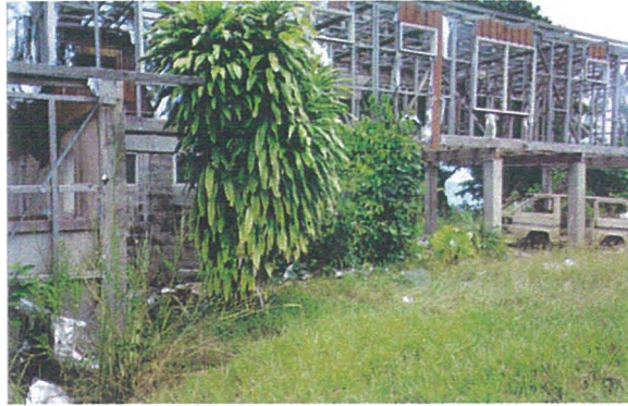
Burnt out house
