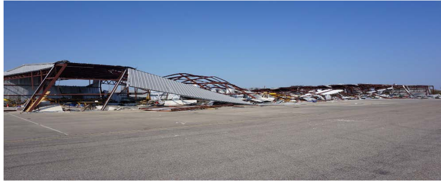
Figure 1 Damaged Hangar Structure at Port Aransas County Airport. Photo taken on September 9, 2017 during GEER reconnaissance trip
