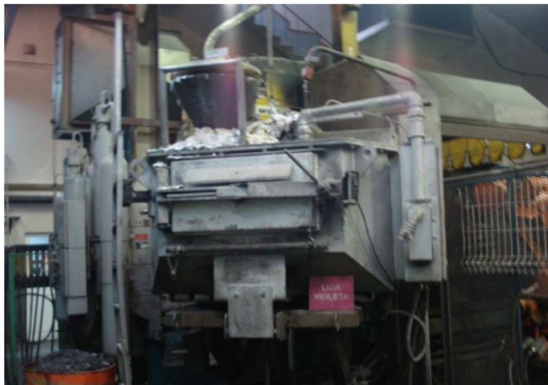
Figure 29 Maintenance Oven in Die-Casting Industry [28]
