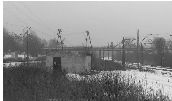
Figure 6. View of the energy installation near the railway viaduct – national road No. 15 over lines No. 353 and No. 281
