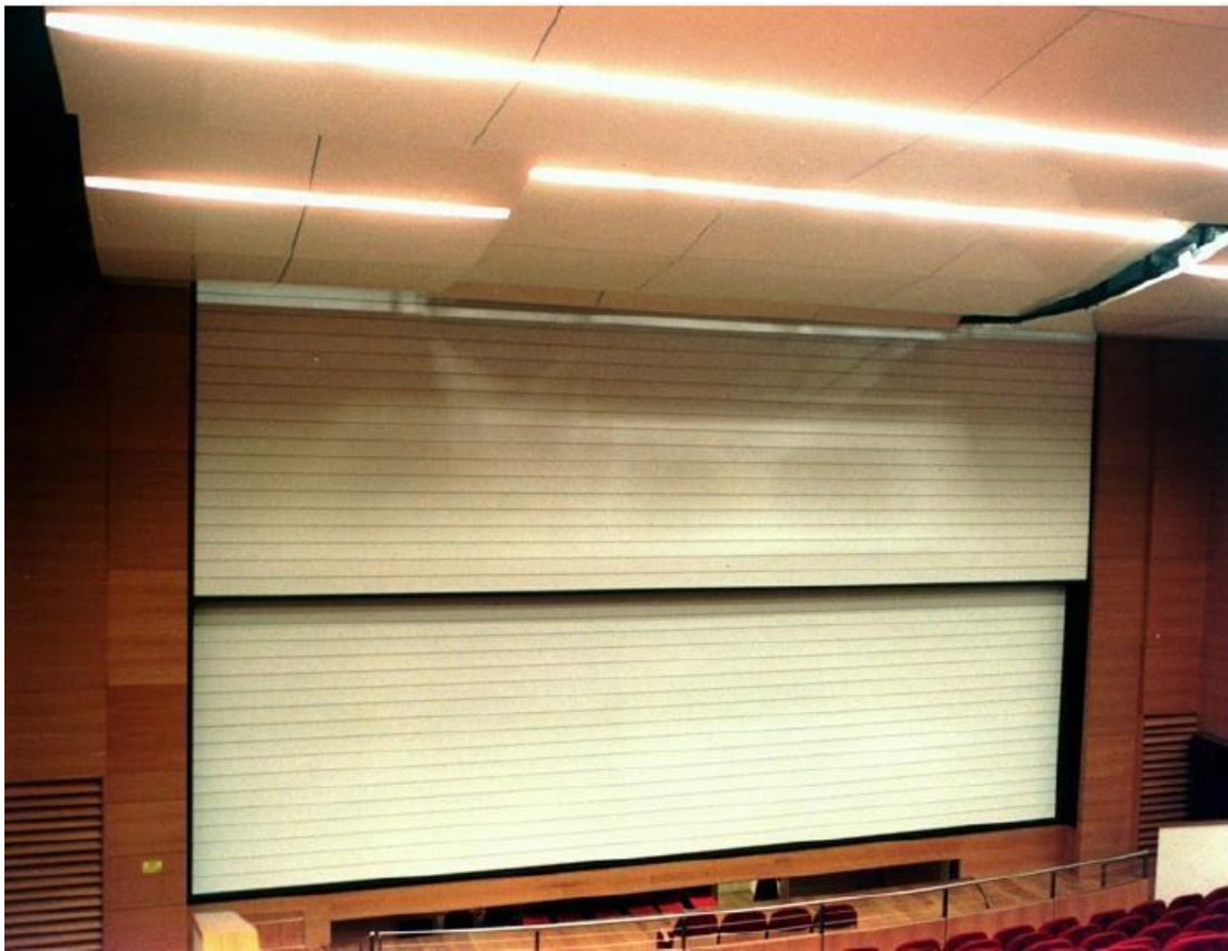
Figure 2. 25 Double leaf fire safety curtain of the "Lorenzo da Ponte" Theater of Vittorio Veneto. Ref; William Paul Gerhard, "Theatre fires and panics: their causes and prevention", John Wiley & Sons, 2009
