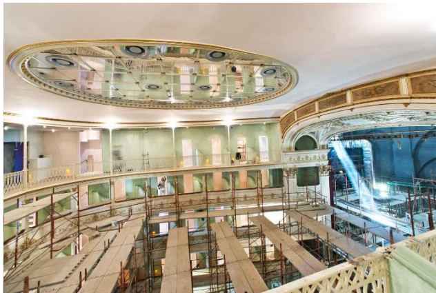
Figure 6.3 Restoration of Niccolini Theater Ref; Available on official site of the Niccolini theater
