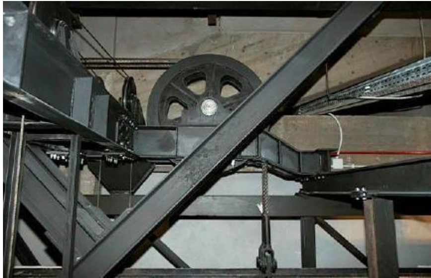
Figure 2. 27 Lifting / lowering system of the fire curtain.
