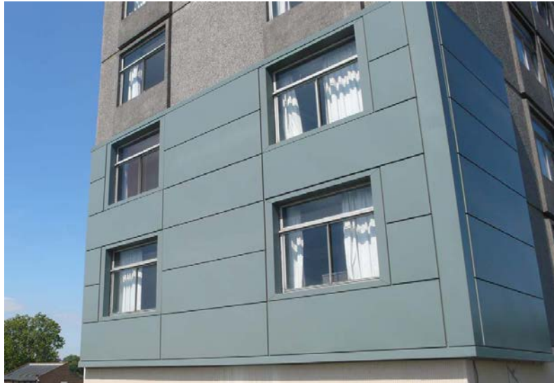
Fig. 3. Building façade with the installed cassette-panels (the perforated panels are the four panels directly between the windows)
