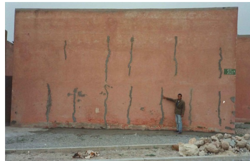
Figure 9. The pattern of vertical cracks identified on the external rammed earth walls of the houses in Mostefa Ben Brahim.
