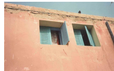
Figure 12. Vulnerability of rendering at the top of an external wall of a rammed earth house in Mostefa Ben Brahim, showing spalling of the rendering.
