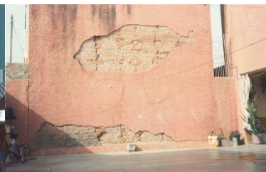
Figure 11. Vulnerability of the roughcast rendering used for the rammed earth houses in Mostefa Ben Brahim. Note the vertical cracks on the wall and black patches at the top of the wall.
