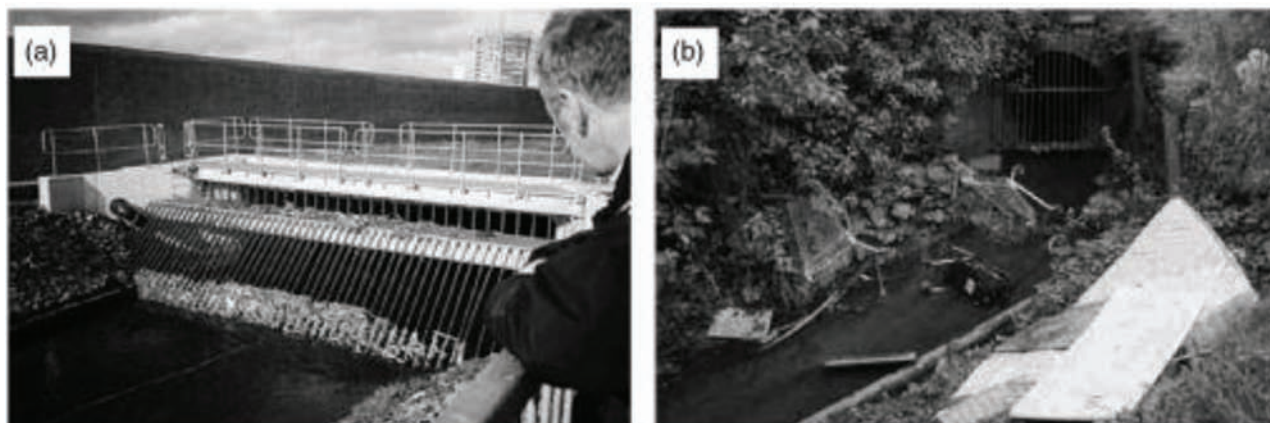
Figure 5.1 (a) Screen protecting inlet to large culvert with leaf-litter accumulation; (b) screen protecting culvert inlet on small channel with fly-tipped waste.
