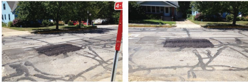
Figure 1.2 Example of a poorly performing utility cut. (Courtesy of Dr. Tommy Nantung and Dr. Jusang Lee, August 2015.)
