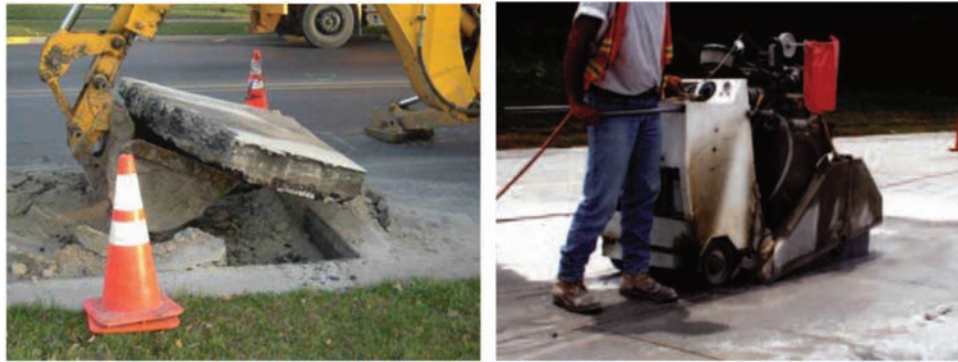
Figure 2.1 Left: asphalt pavement removal (Schaefer et al., 2005); right: saw cutting of a concrete pavement (ACPA, 2009).
