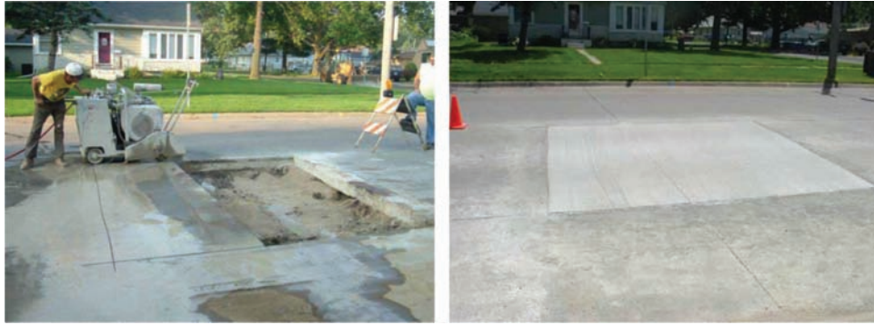
Figure 1.1 Example of a utility cut repair operation on a concrete pavement (Schaefer 2005).
