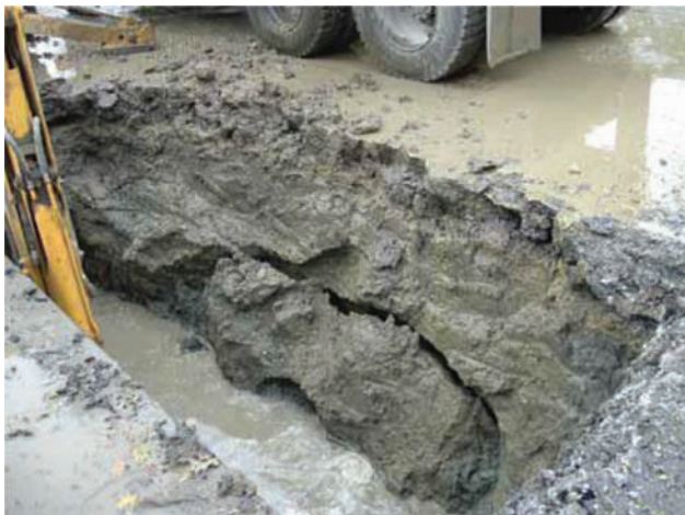
Figure 2.3 Material sloughing off the edges of a trench (Schaefer et al., 2005).
