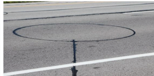
(c) Inductance loop at WIM station
