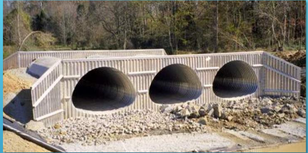
Corrugated Metal Arch
