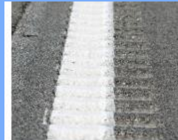
Example of an edge line rumble stripe.
