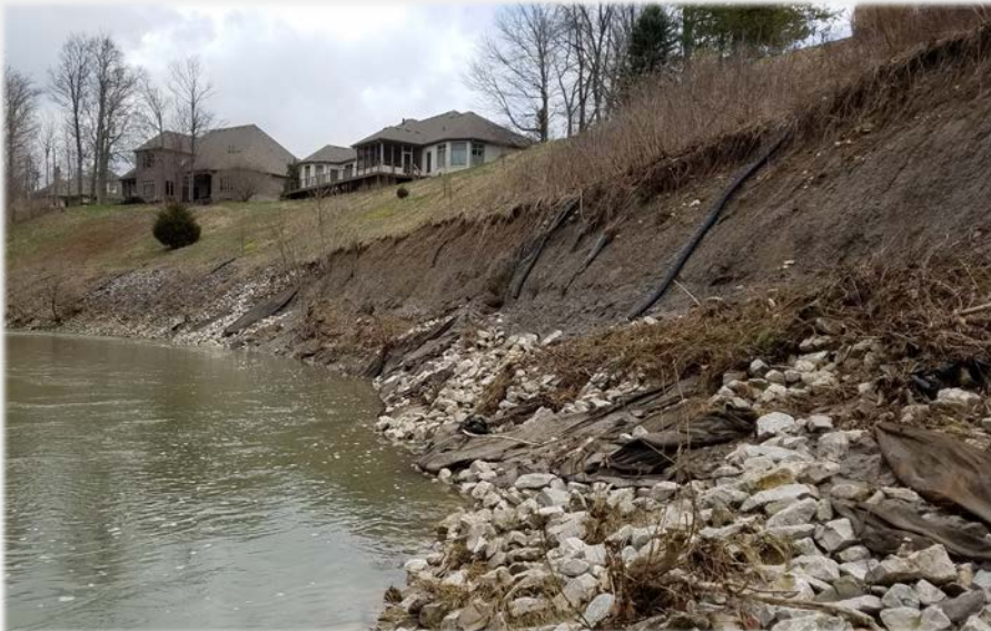
Lack of maintenance/management results in slope failure White Lick Creek in Avon, IN
