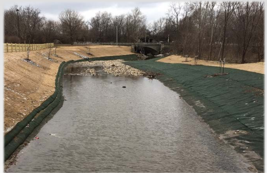
Robust materials protecting critical infrastructure in a flashy stream Bean Creek in Indianapolis, IN
