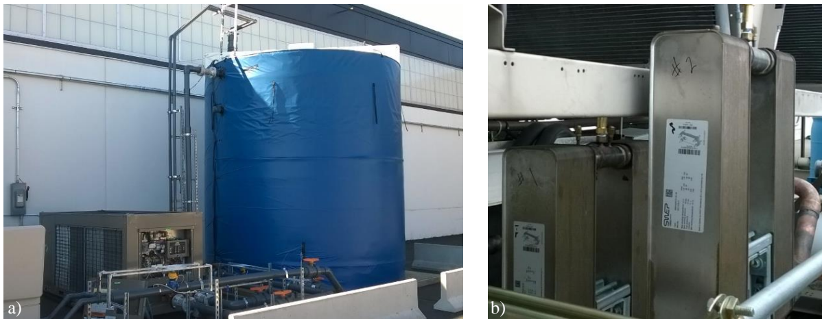
Figure 2: ITESS: a) supplemental chiller and water storage tank; b) sub-cooler plate heat exchangers
