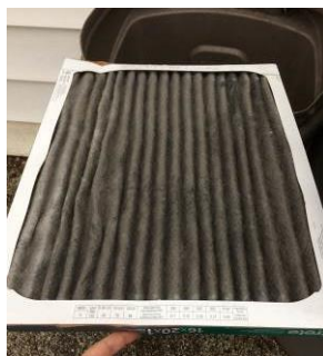
Figure 2: Dirty air filter to be replaced
