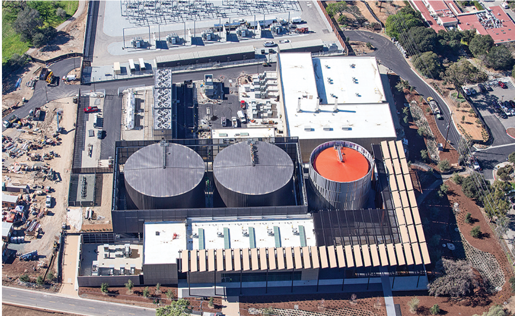
Figure 2: The new heat-recovery system to provide heating and cooling to the campus constructed as part of the $485-million Stanford Energy System Innovations (SESI) project Blair (2016).
