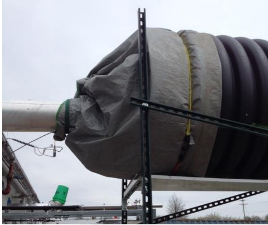
Figure 4.12: Seal between Inlet Ducting and Settling Chamber.
