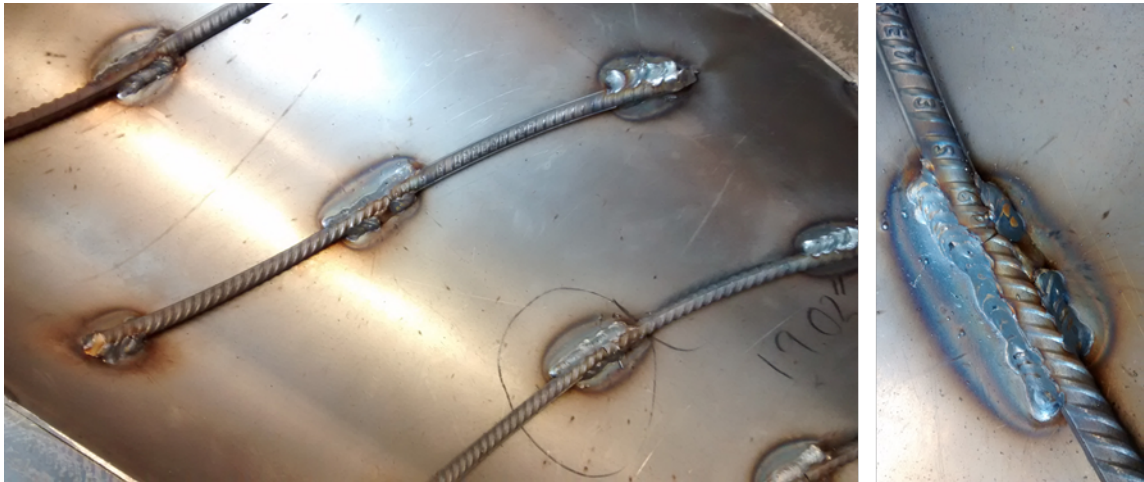
Figure 17 - The upper concave with pieces of rebar placed in a helical form. Left: the arrangement of the pieces. Right: the welds holding the pieces to the concave. Source: Author.
