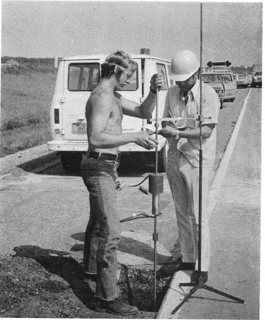
Figure 5. A low-load penetrometer is being used to test the subgrade of an interstate highway. The drop hammer is in the midst of its free fall. The note taker records an initial and final scale reading at the pointer and, by subtraction, determines the millimeters of penetration of the cone point.
