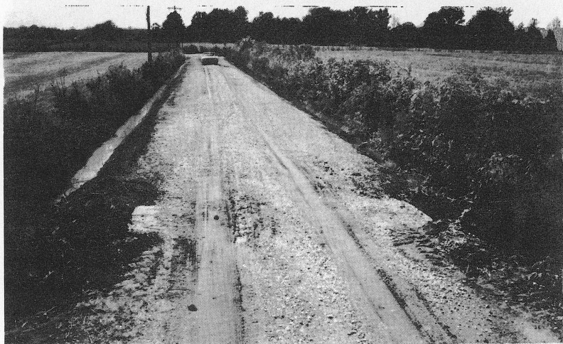
Fig. 18. This ditch illustrates two weaknesses—the outlet is plugged with debris, and the slope is too flat. Even when the outlet is cleaned out, this ditch will need more slope to drain all the water.
