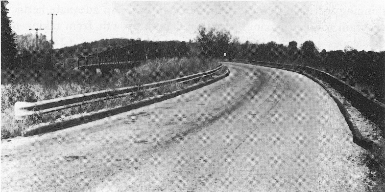
Fig. 14. Asphalt curbs contain water in this roadway, carrying it away from the structure and steep slopes.
