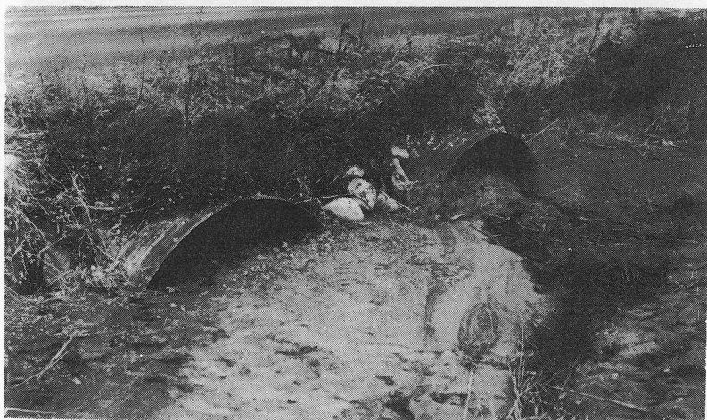
Fig. 25. This culvert is almost completely useless until it is cleaned out and the erosion which produced the silt is stopped.
