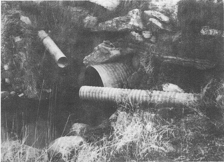
Fig. 22. Two pipes overhanging the stream provide outlets to the ditch from both sides of this stream.
