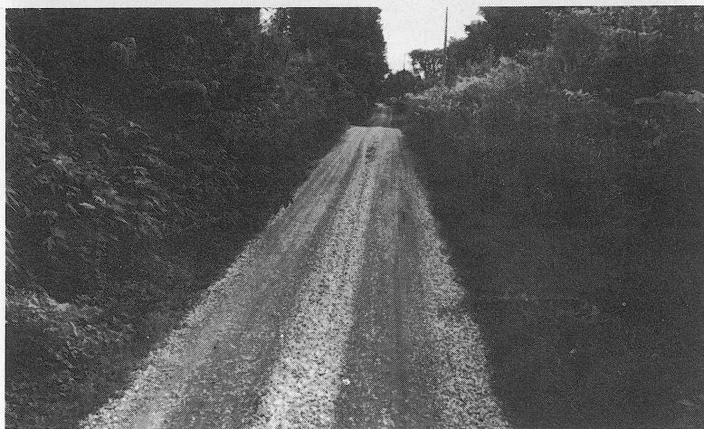
Fig. 26. Two extremes—above, a well constructed and maintained ditch; below, a ditch completely overgrown with weeds and brush.
