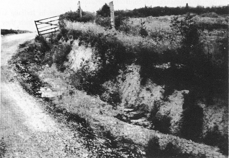
Fig. 1. A flatter cut slope would improve sight distance and establishment of vegetal cover.
