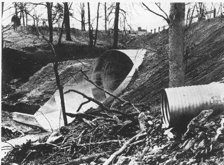
Fig. 35. Two end treatments are illustrated here. Note the smaller pipe extended straight beyond the toe of the embankment, and the larger pipe beveled to fit the slope. A concrete sill at the invert of the large pipe prevents undermining. (Courtesy Armco Drainage and Metal Products, Inc.)
