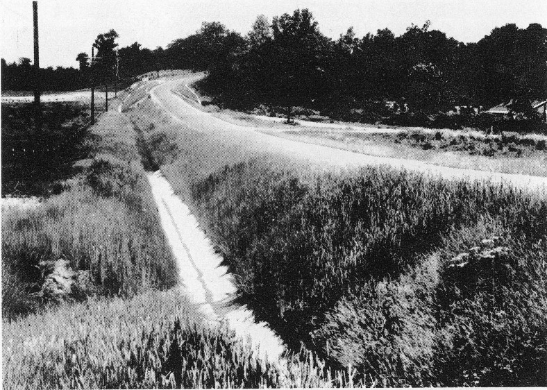
Fig. 7. Application of the principles of slope protection is well illustrated on this county road. Note the flat slopes with well rounded edges, and the turf cover over the entire slope.
