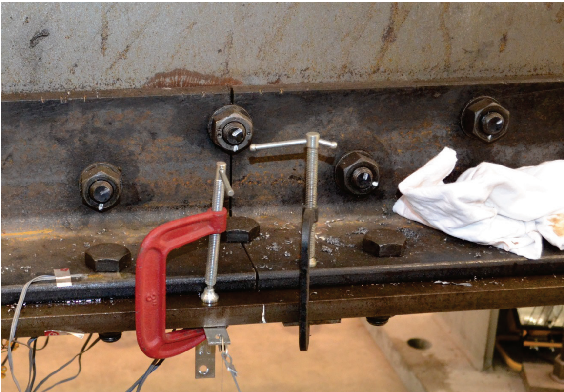
Figure 3-63 Specimen 46-5 severed flange angle
