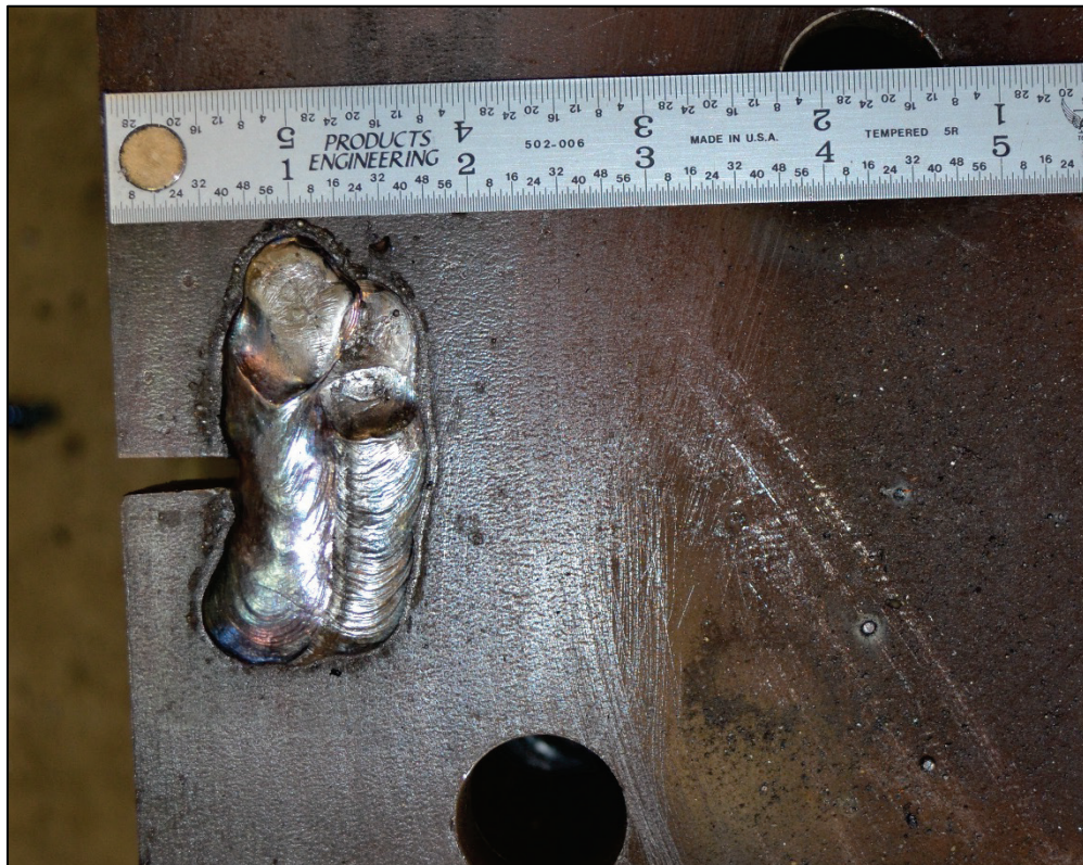
Figure 3-24 Edge notch with Wearshield ME weld at notch tip
