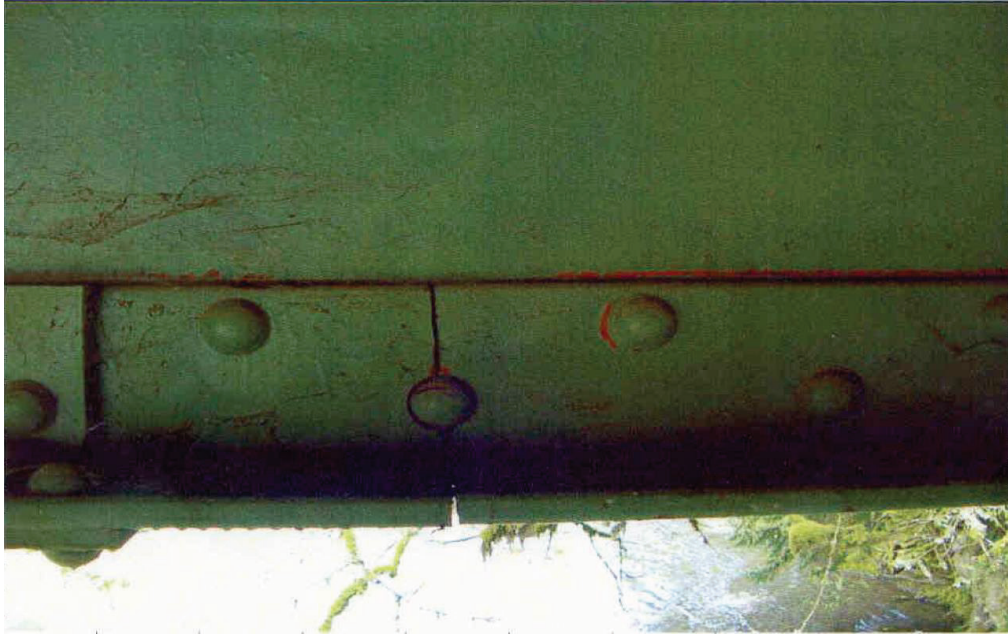
Figure 2-2 Interior view of fractured flange angle (Lovejoy, 2001)
