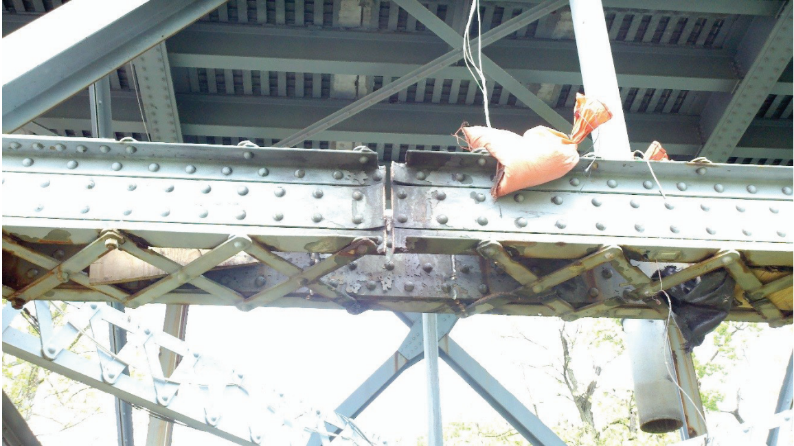
Figure 2-9 Partially severed bottom chord, Milton Madison Bridge approach span
