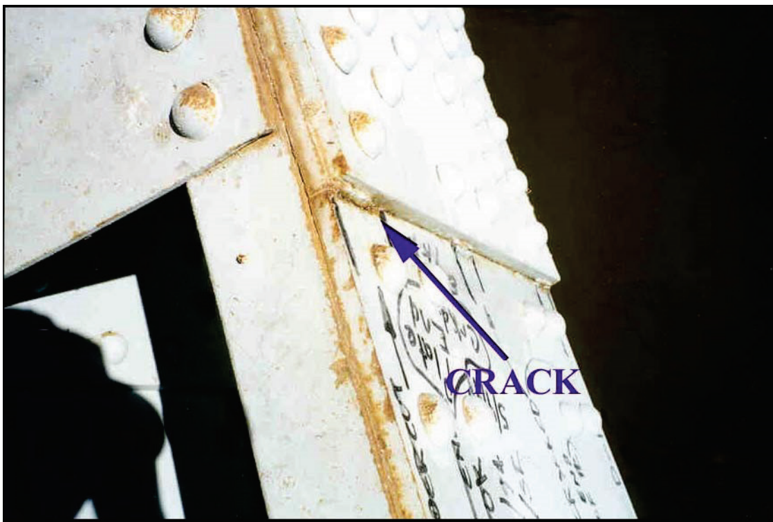
Figure 2-6 Fractured tie girder plate, Hastings Bridge (Niemann, 1999)
