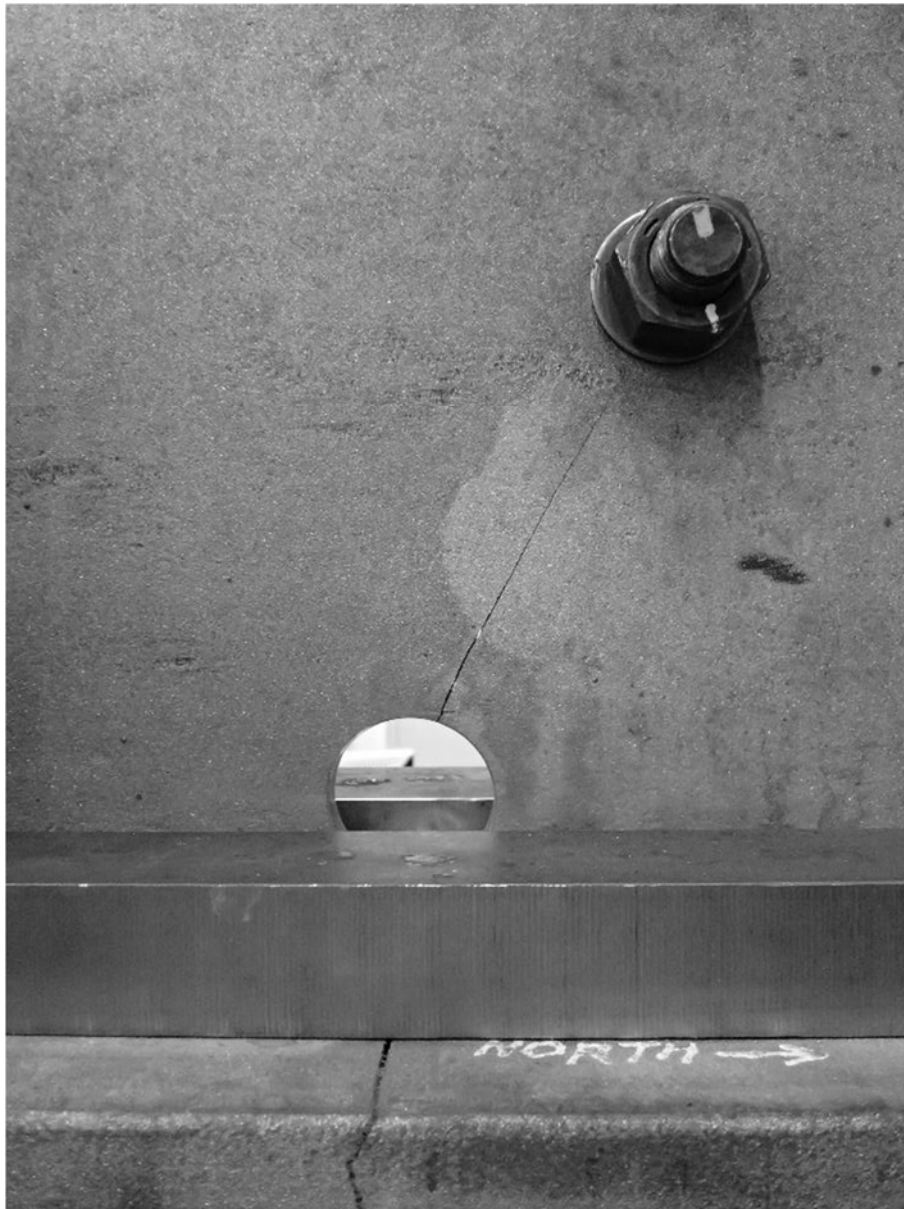
Figure 3.14: Open and Bolted Crack Arrest Holes at a Failed Cover Plate
