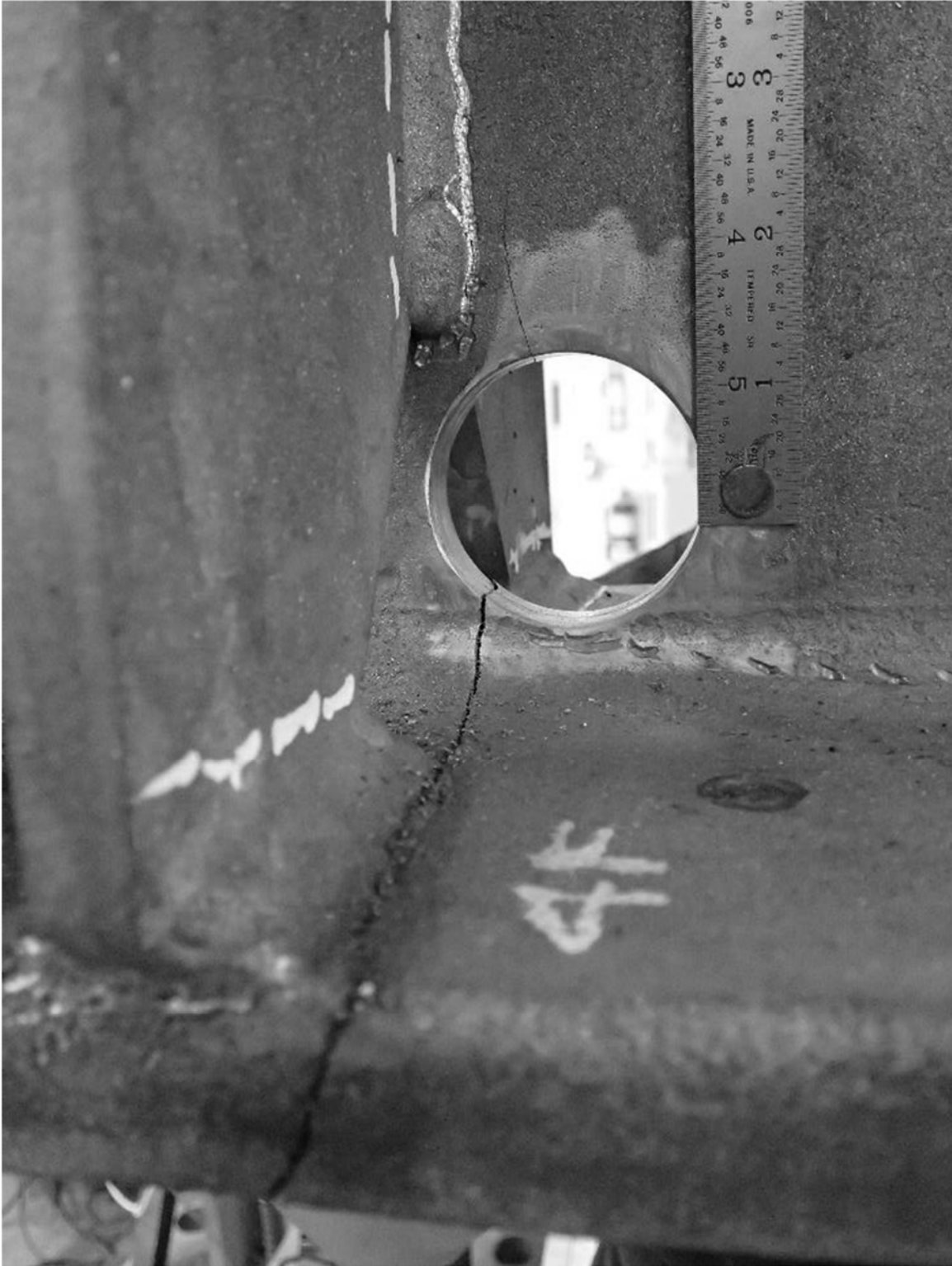
Figure 4.1: Fatigue Crack Initiated from Transverse Stiffener Weld Toe
