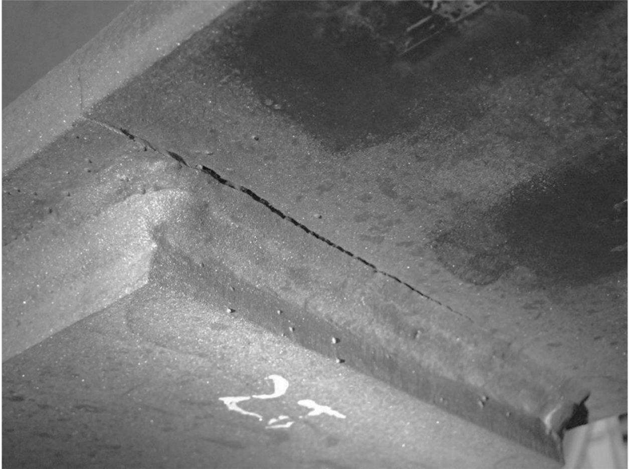
Figure 4.2: Fatigue Crack Initiated from as-welded Cover Plate Weld Toe
