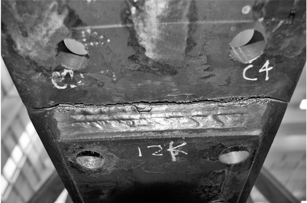
Figure 4.3b: Fatigue Crack through Weld Toe of Treated Cover Plate Weld
