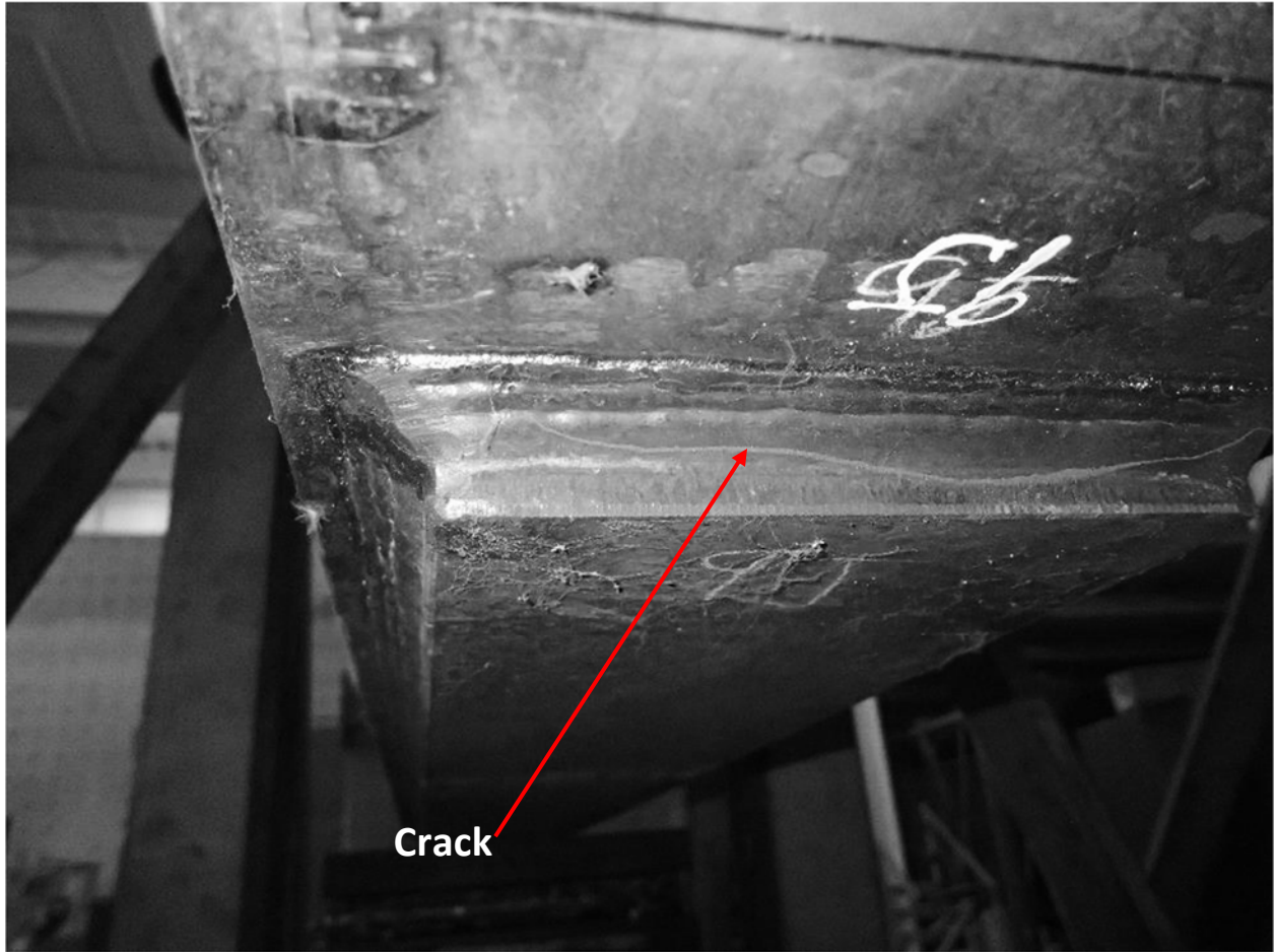
Figure 4.3a: Fatigue Crack through Weld Throat of Treated Cover Plate Weld
