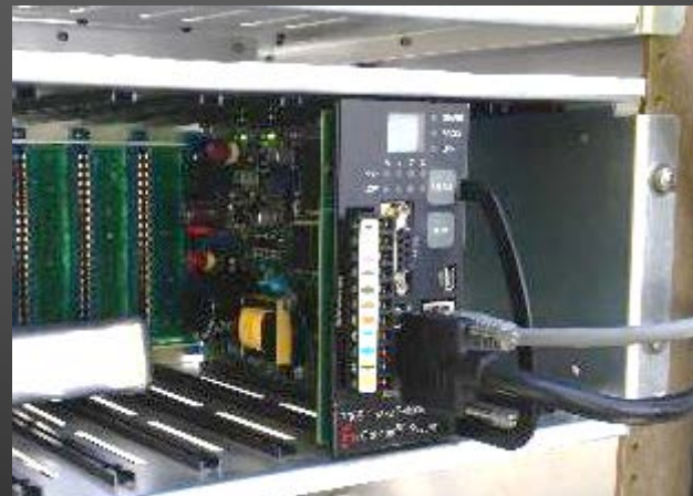
Verify Phase Selector Configuration
