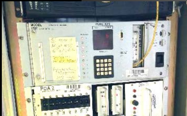
Verify TSP Configuration in Traffic Controller
