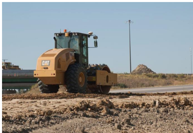
FIGURE 1 PADFOOT VIBRATORY SOIL COMPACTOR USING MDP TECHNOLOGY ON COHESIVE SOILS – IOWA USA
