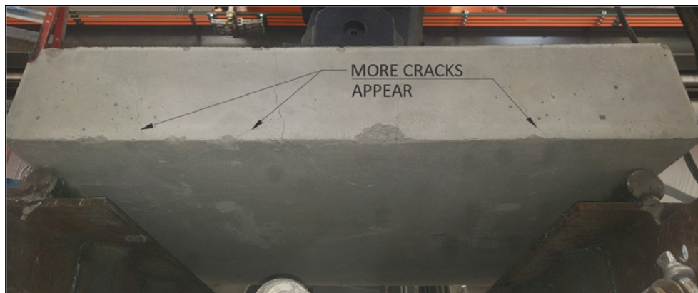
Figure 5-6 Load was increased to 9,000 lbs. (approximately 20,000 cycles)
