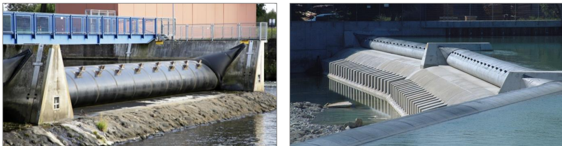
Figure 1. Weir sills at rubber gates: Marklendorf, Germany (left) and Ebenhofen, Germany (right).
