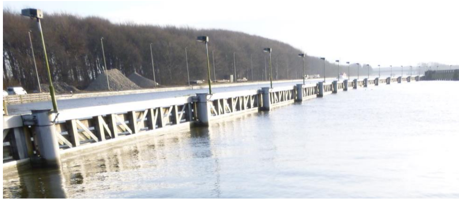
Figure 6. Picture of the guiding structures between the Middle Lock and the Push Convoy Lock. Picture: Jenna Vergeynst.
