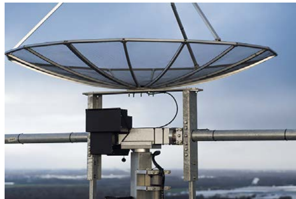
Figure 6: S-band Ground Station Upgrade
