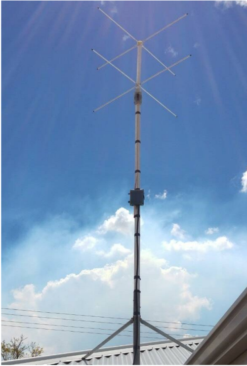
Figure 14: Omnidirectional antenna for Rick Zathras' ground station #23 in Perth, Australia.
