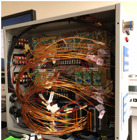
Figure 3 ACCS Electronics Box
